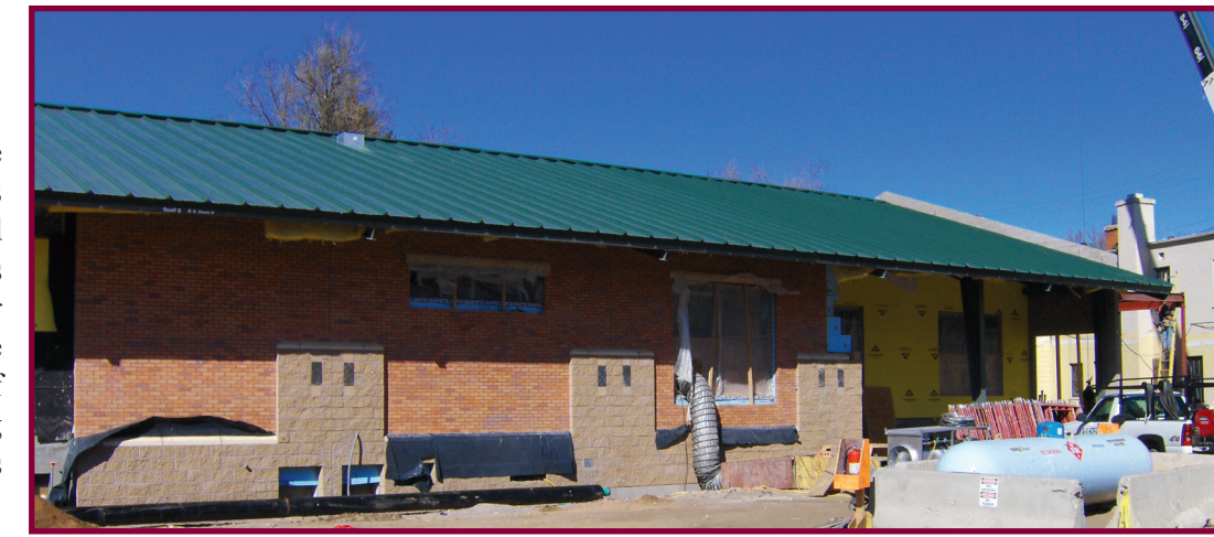
Progress to date on The New Marian House dining hall and kitchen. Scheduled to open in May 2008.
